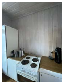
Manglende ventilering over kokesone.
