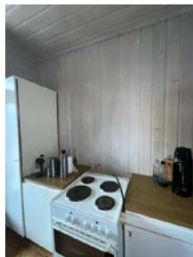
Manglende ventilering over kokesone.
