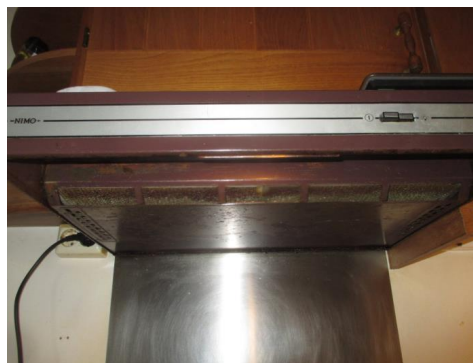
Noe eldre ventilator.
