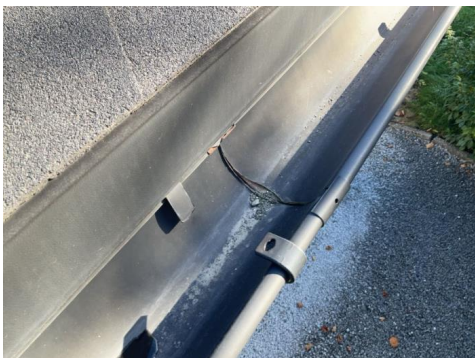
Rust i takrenner.
