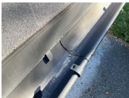
Rust i takrenner.
