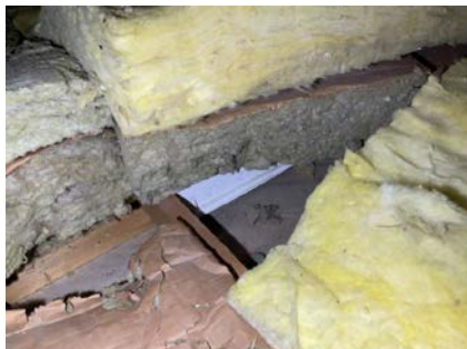
Manglende tetting rundt spotkasser.
