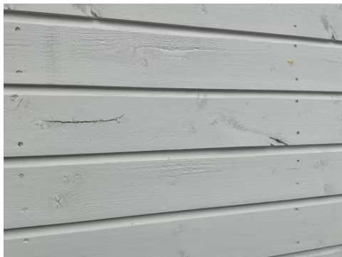
Sprekker i panel.
