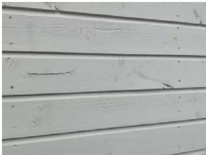
Sprekker i panel.
