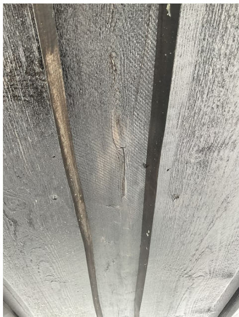
Sprekker i panel.
