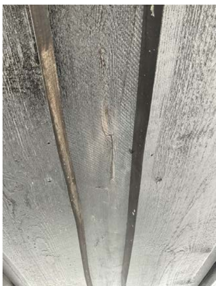
Sprekker i panel.
