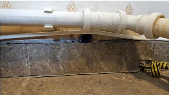
Glippe i fuge i overgang gulv/vegg.
