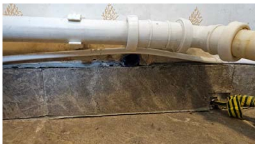
Glippe i fuge i overgang gulv/vegg.
