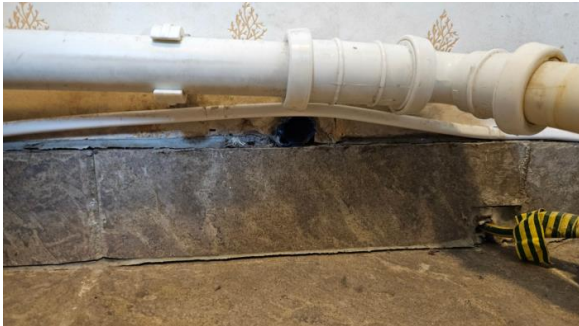
Glippe i fuge i overgang gulv/vegg.
