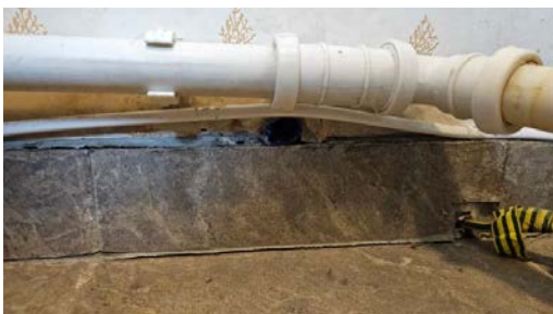
Glippe i fuge i overgang gulv/vegg.
