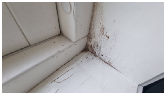
Fuktsvell i vindusforing.
