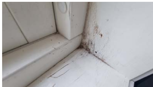
Fuktsvell i vindusforing.
