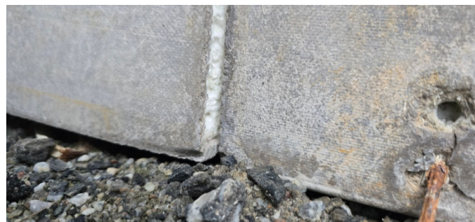
Sprekker i ringmurselement
