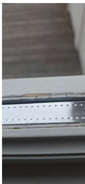
Sprekker i gummilister inn mot glass
