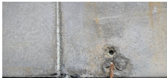
Sprekker i ringmurselement
