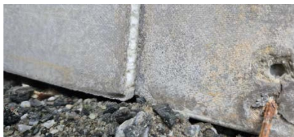
Sprekker i ringmurselement
