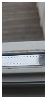
Sprekker i gummilister inn mot glass
