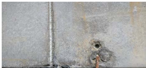
Sprekker i ringmurselement
