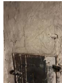
Riss/sprekker i pipe/mur over feieluke.
