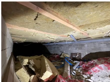
Manglende plater under bjelkelag
