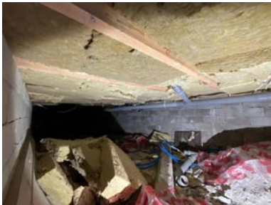
Manglende plater under bjelkelag
