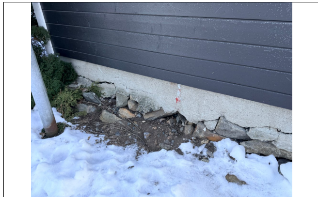
Fundament bod, masser raser ut.
