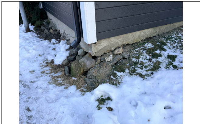
Fundament bod, masser raser ut.
