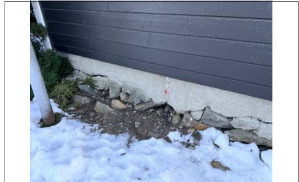
Fundament bod, masser raser ut.
