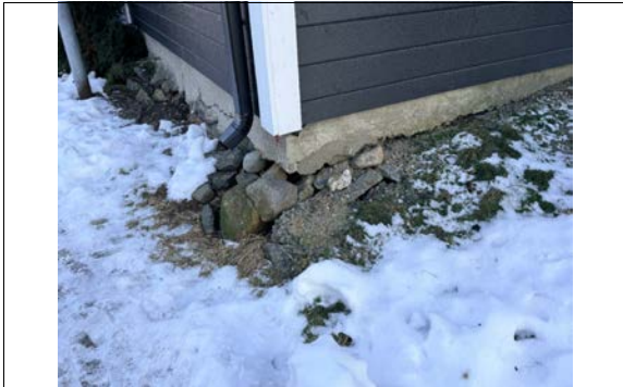
Fundament bod, masser raser ut.
