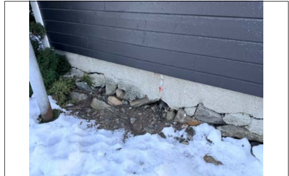
Fundament bod, masser raser ut.
