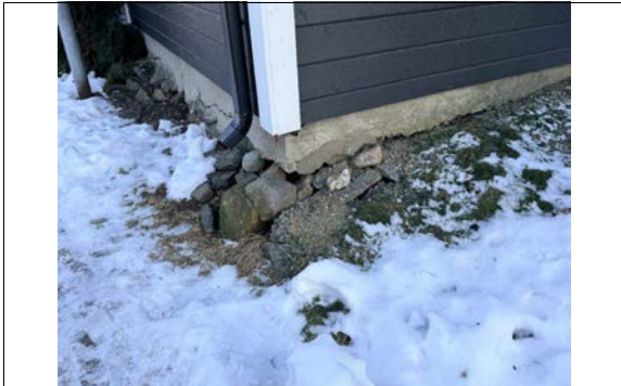
Fundament bod, masser raser ut.
