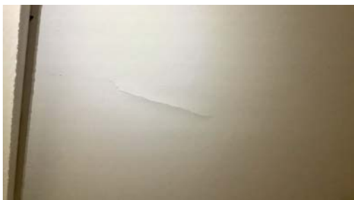
Oppsprekking i himling.
