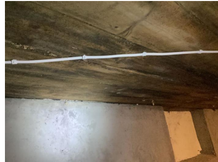
Misfarging i himling.
