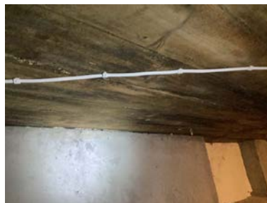
Misfarging i himling.
