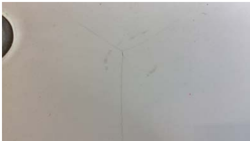
Riss i servant.
