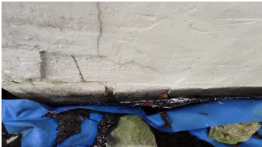
Grunnmursplasten mangler klemlist.
