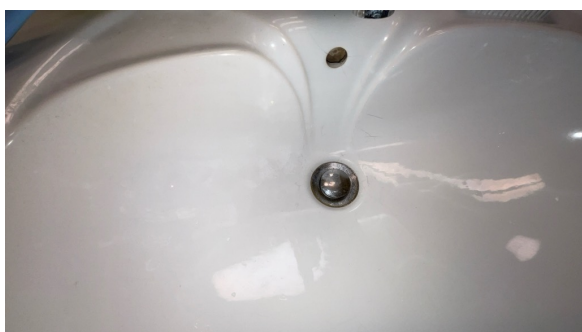
Riss i servant
