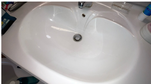
Riss i servant
