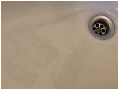
Krakelering i overflate i vask.
