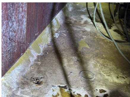
Behov for rengjøring under kabinett
