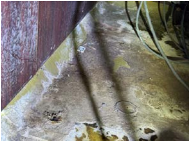
Behov for rengjøring under kabinett
