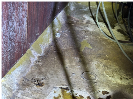
Behov for rengjøring under kabinett
