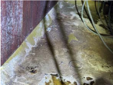
Behov for rengjøring under kabinett
