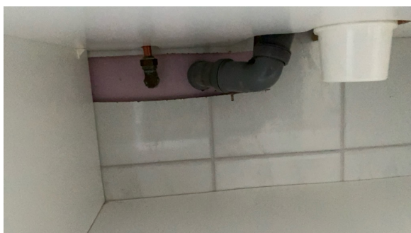
Hull i baderomsplate under vask
