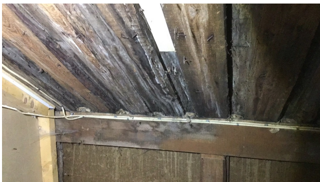
Fuktskader i undertak i kott
