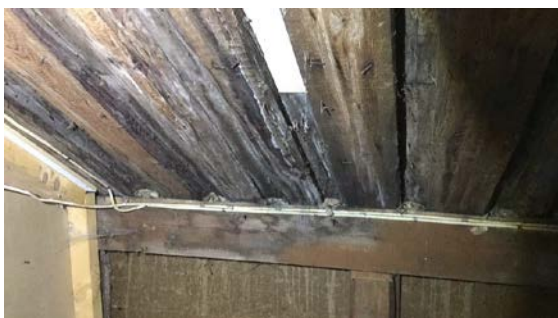
Fuktskader i undertak i kott
