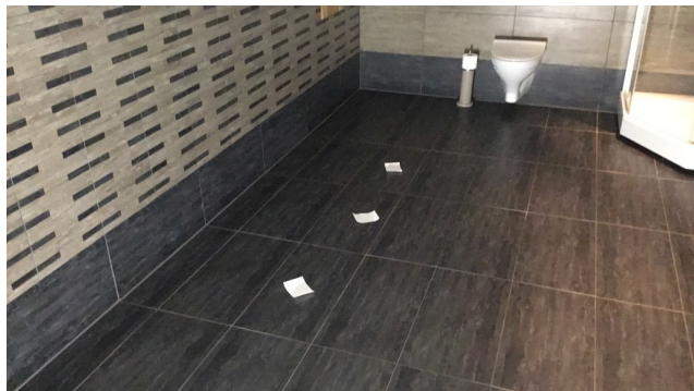
Hulrom under 3 fliser
