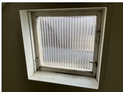
Sprekker i glass.
