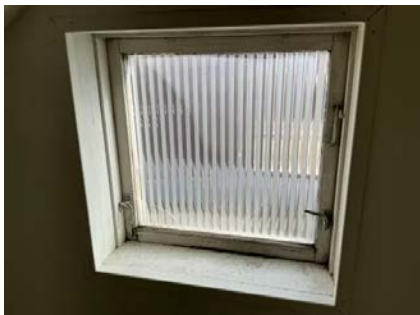
Sprekker i glass.
