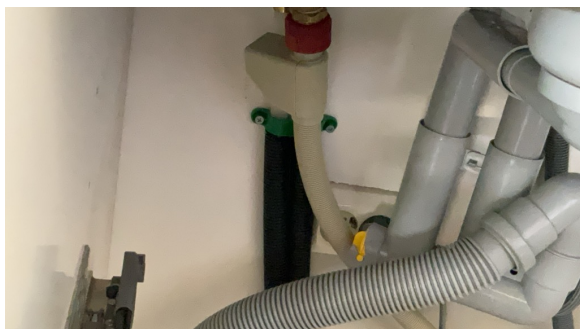
Tettemuffer mangler under kjøkkenbenk
