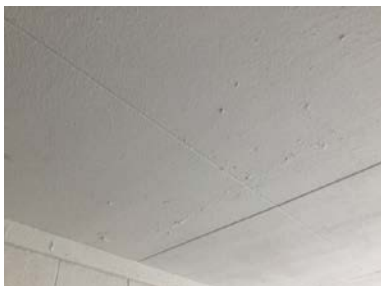
Grov overflate i himling.
