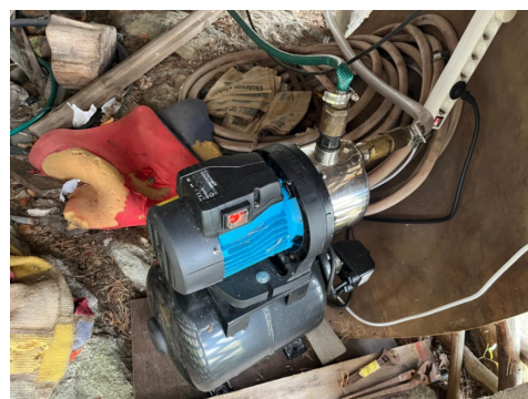
Vannpumpe under veranda.
