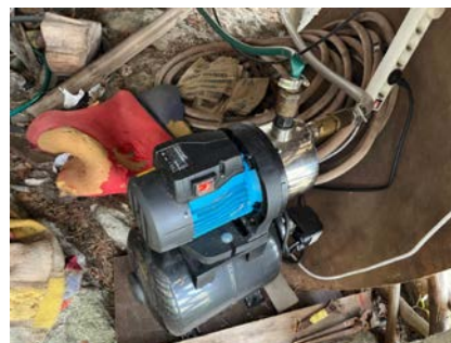
Vannpumpe under veranda.
