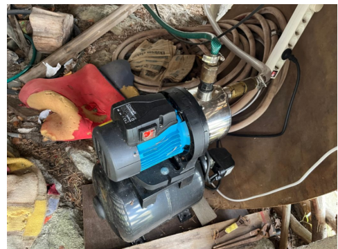
Vannpumpe under veranda.
