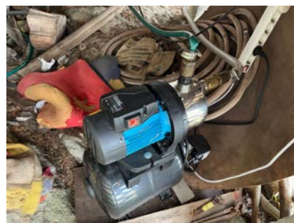
Vannpumpe under veranda.
