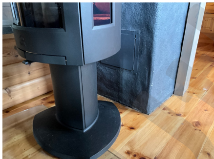
Mangler ubrennbar plate bak ovnen under feieluke.
