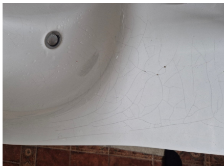
Krakelering i servant.
