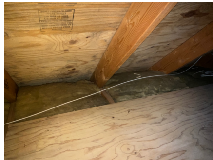
Fuktmerker i undertaket.
