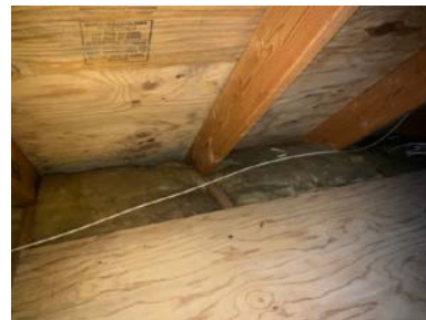
Fuktmerker i undertaket.
